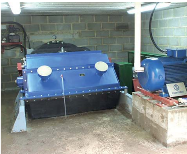
Figure 1.2 The newly installed crossflow turbine at Alport Mill (photo courtesy of Derwent Hydro)
