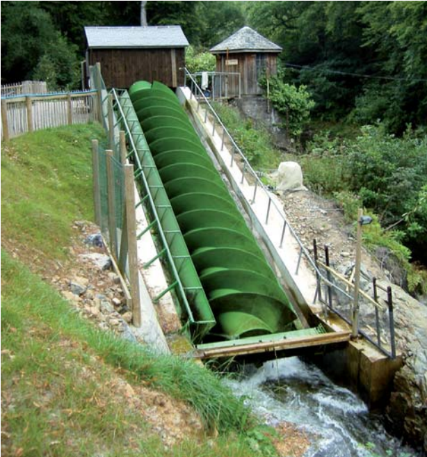
Figure 2.7 Screw at River Dart Country Park, Devon (photo courtesy of MannPower)
