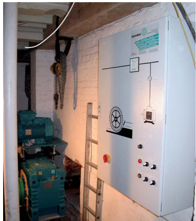
Figure 4.5 Control panel at Lemsford Mill, Hertfordshire (photo courtesy Ramblers Worldwide Holidays)
