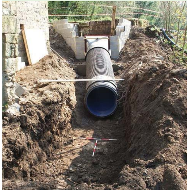
Figure 3.1a/b Burying the pipe ('penstock') carrying the water from the intake to the powerhouse at Alport Mill, Peak District (photos courtesy of Derwent Hydro)
