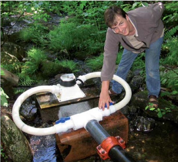
Figure 2.13 A DIY pico hydro installation in Canada
