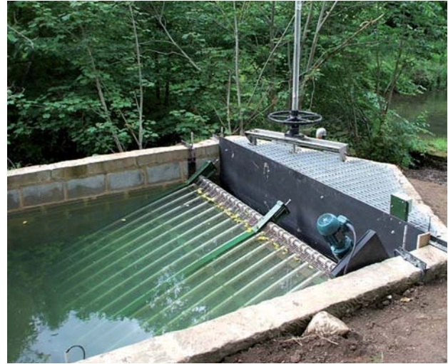
Figure 2.16 Band screen at Alport Mill, Peak District (courtesy of Derwent Hydro)
