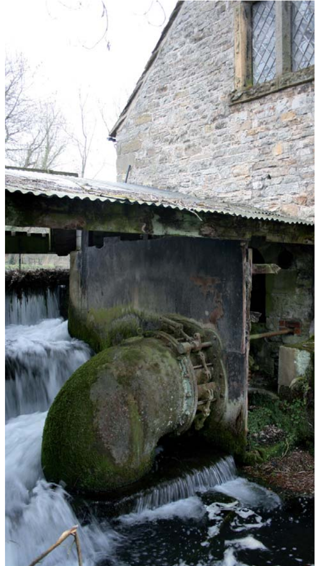
Figure 2.12 An original Francis turbine in situ at Flewitt's Mill, Ashford in the Water
