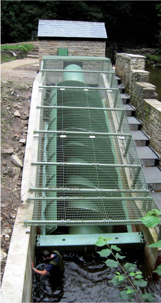
Figure 1.1 The Torrs Hydro Archimedes screw at New Mills in High Peak (photo courtesy of MannPower)
