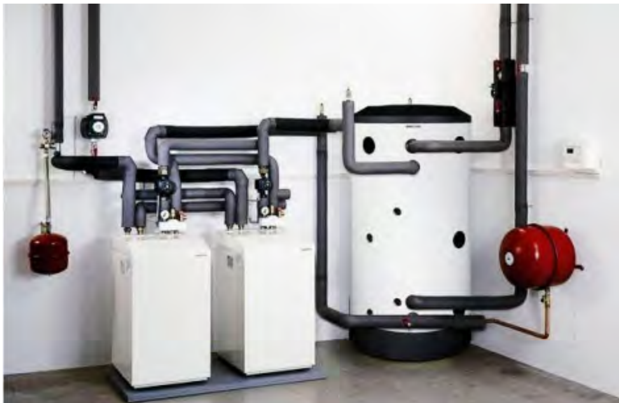
Above, a Stiebel Eltron WPW44 heat pump installed in a plant room with a buffer tank (heat store).
