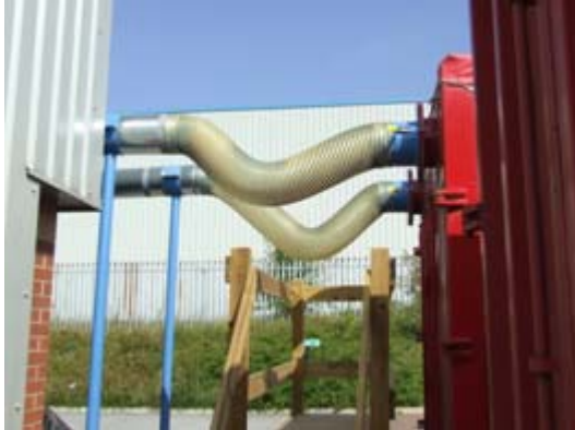
Left, Central Joinery's wood dust handling system.
