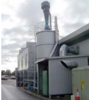
Left, Central Joinery wood dust handling system, storage silo, and burner.
